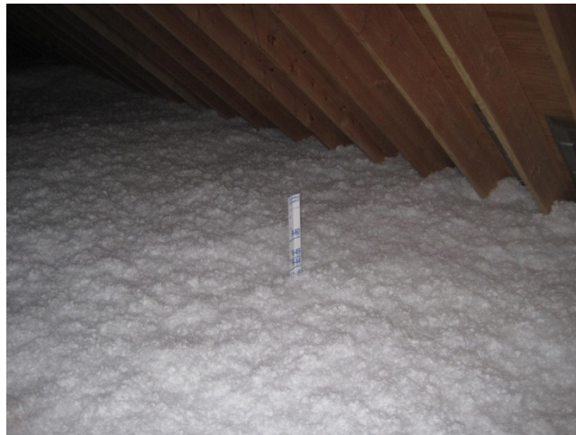
Figure B-15: Grade I Blown Fiberglass—Attic
